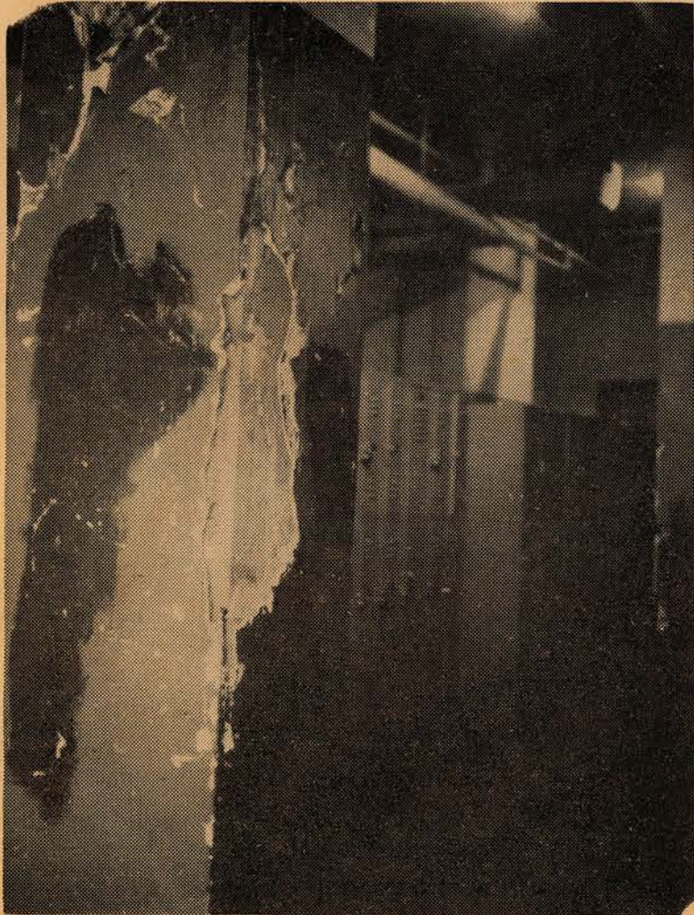
PICTURE TELLS STORY: CRUMBLING PLASTER
