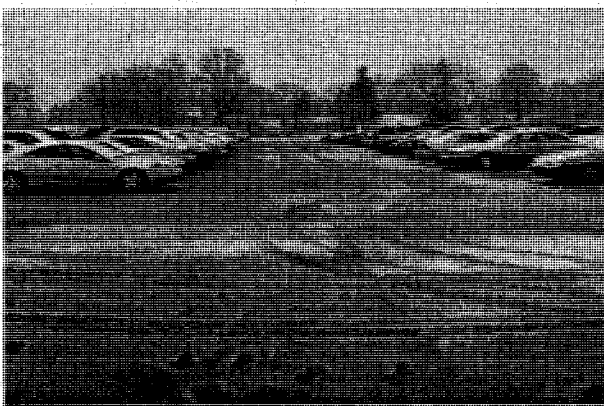
Recent incliment weather shows SHS parking lot at it's worst
