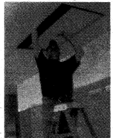
A member of the maintenance crew feeds electrical cable through the ceiling of the hall.
