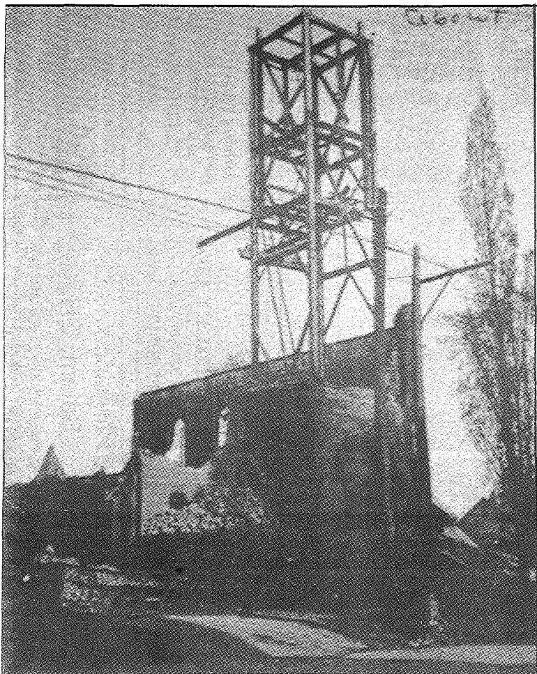
The skeleton of the bell tower juts upward in this 1909 photo taken when the Salem Methodist Church was torn down to make way for a new building.
