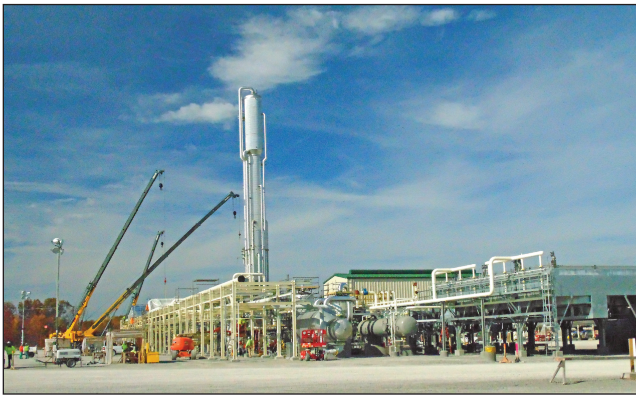
The tallest part of the Hickory Bend Cryogenic Processing Plant in Springfield Township is the demethanizer tower which separates liquid natural gas, vapors and water from oil and gas sent to it from area wells. Applying temperatures from -100 to -150 degrees below zero separates methane which is "pulled off the top," according to engineer Scott Singer. He said traces of ethane may also be produced. (Salem News photos by Larry Shields)
