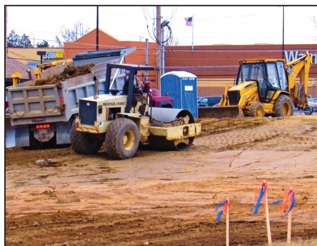
Crews from Less Contracting of Salem are shown trucking in fill dirt to the site of the Holiday Inn Express on Thursday afternoon. They were loading the dirt from behind the Home Depot store.
