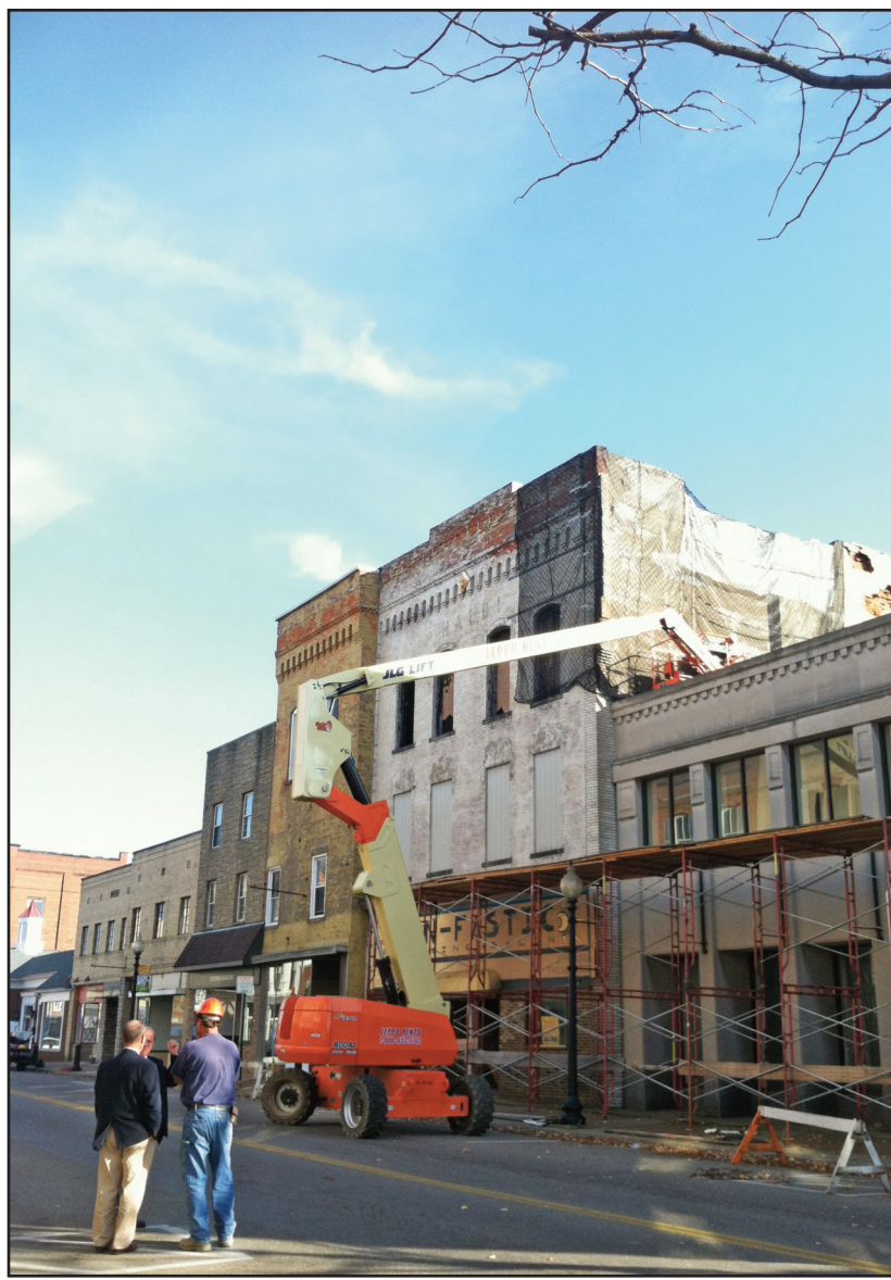
Salem City Service/Safety Director Ken Kenst, Mayor John Berlin and a worker on the TanFastic fix project watch as another worker for Siitle Construction finishes securing the netting on the west side wall Monday afternoon. State Street was expected to reopen sometime this morning after an engineer inspects the work, which was delayed for a short time due to a small fire workers extinguished after seeing smoke. The Salem Fire Department used a thermal imaging camera and found no additional hot spots. (Salem News photo by Mary Ann Greier)
