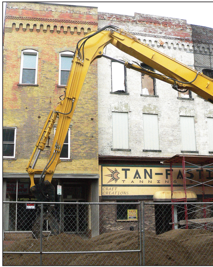
The claw of an excavator rests in front of the TanFastic building and the former Rosetti Bakery building to the left, awaiting the start of the TanFastic demolition on Monday. City council gave Mayor John Berlin permission to make an offer to buy the Rosetti building owned by the Soltis family in hopes of demolishing two buildings for the price of one. (Salem News photo by Mary Ann Greier)
